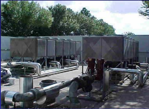
New Energy Efficient Chillers at Public Works
