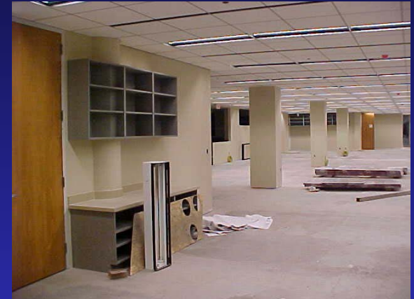
New energy efficient lighting at the Administration Center
